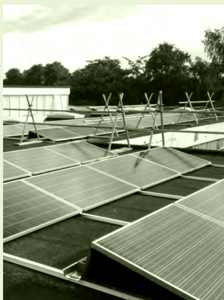
Image: Morgans Primary School Solar Panels (source: Hertford Energy Now)
