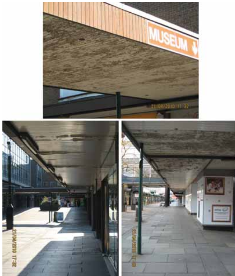
Examples of poor maintenance
