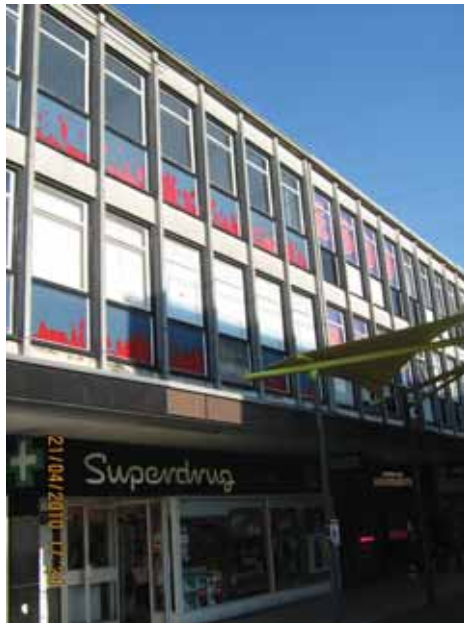
Poorly maintained building frontages
